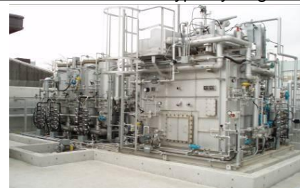
Reformers at off-site type hydrogen station
